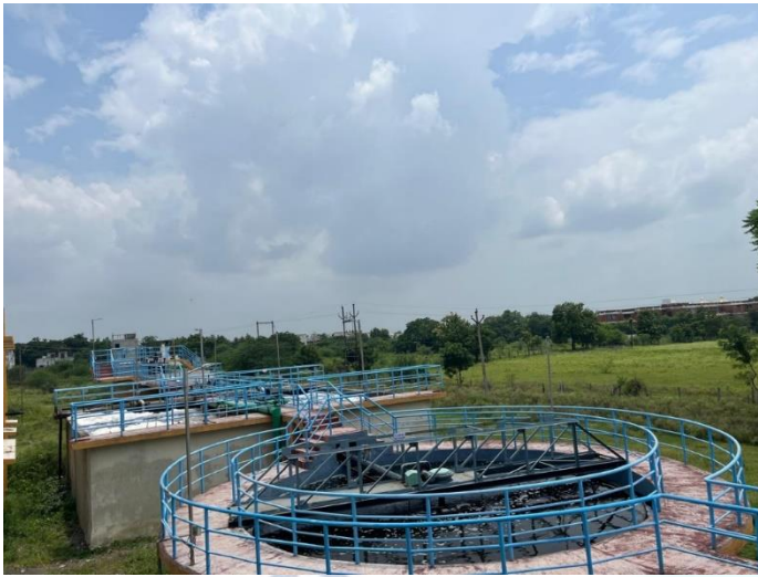
Fig.3.3: 3.5 MLD STP based on MMBR
