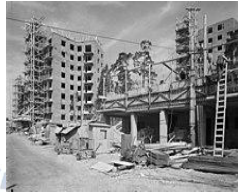
The first residential houses built with Slip forming, was erected 1950 in Västertorp.
