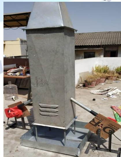
Plate 9 Cooling Tower Unit
